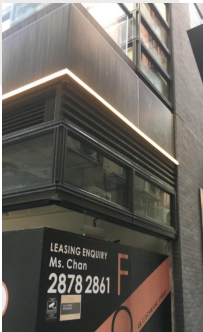
Exterior LED Strip with Control and Metal Cladding
